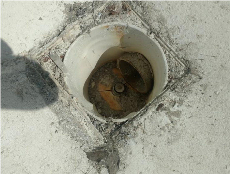
Figure 2-16: Pool Main Drain Failure
