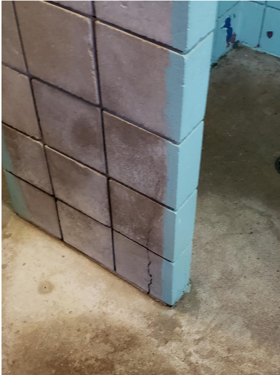
Figure 2-9: Cracking in The Bathhouse Wall
