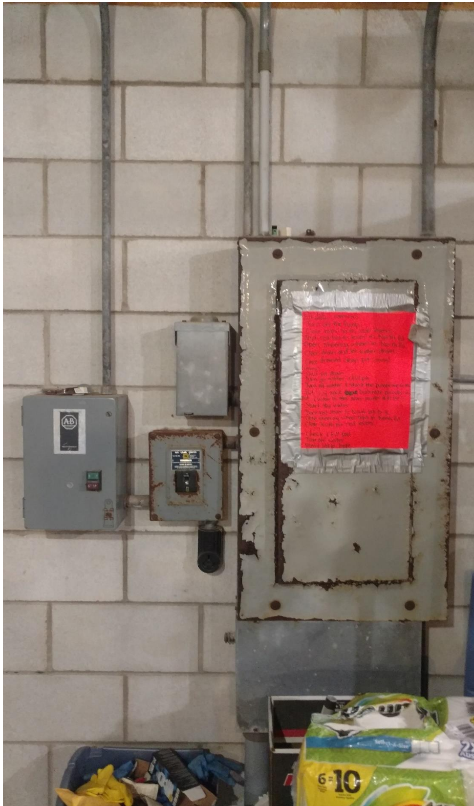
Figure 2-13: Electrical System Condition
