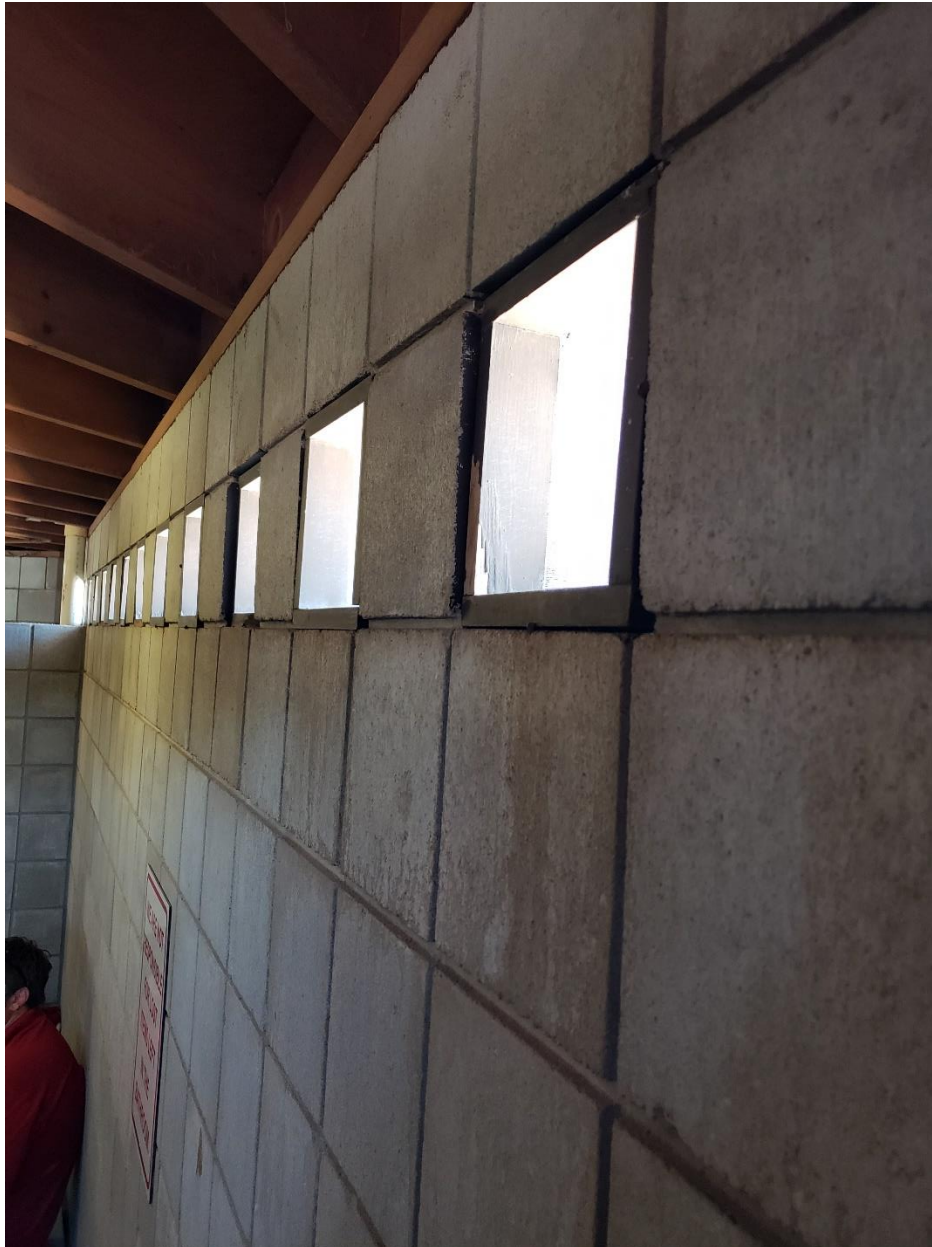
Figure 2-6: Locker Room Ventilation
