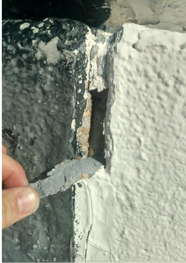
Figure 2-15: Pool Joint Failure
